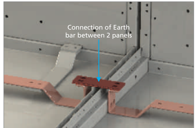
Figure 4.6 C Earth Bar View after Connection
